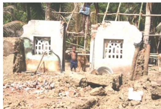
A home destroyed
